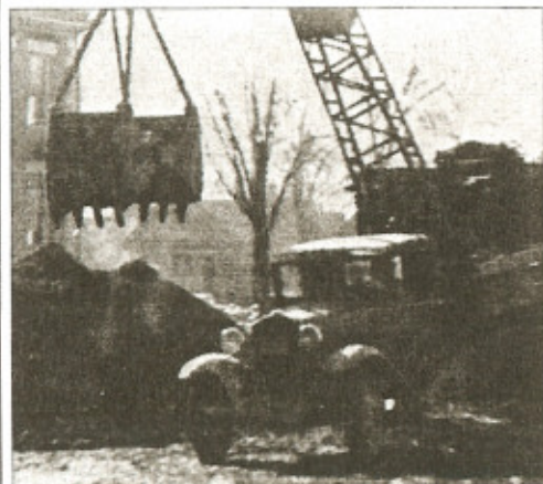
A crane lifts portions of the frame for what is now known as Changnon Gymnasium on the campus of Mt. Vernon Township High School. SUBMITTED PHOTO
